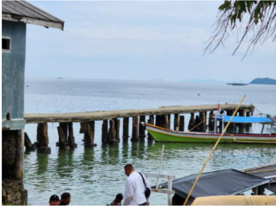
Figure 1 Degradation of concrete columns, beams, and plates at Way Ratai pier, Lampung, Indonesia.
