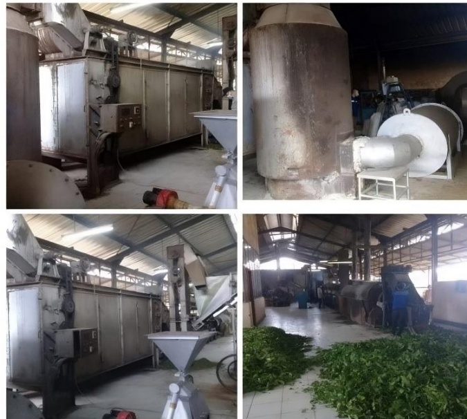
Figure 7. A set of tea dryers consisting of cyclone burners, hammer mills, jaw crushers and heat exchangers (BBPMBTekmira, 2021)
