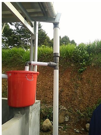
Figure 2. Centrifugal System Installed in Rainwater Harvesting
