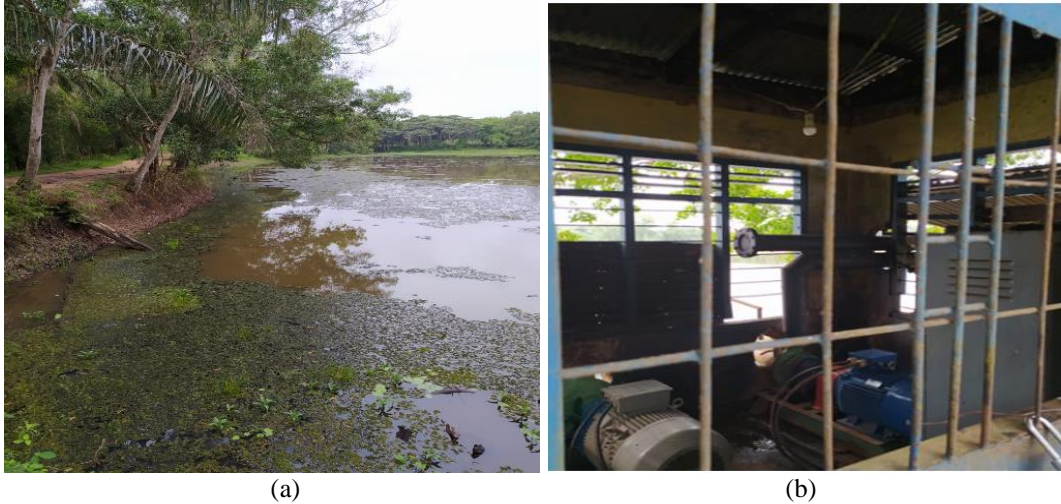
FIGURE 3. (a) One of pond location where silting occurs due to sedimentation. (b) The water pump used to drain water from the pond to factory.
