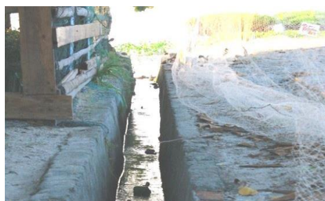
Fig 4. Drainage system in Pramuka island, the surface runoff directly to the sea 36
