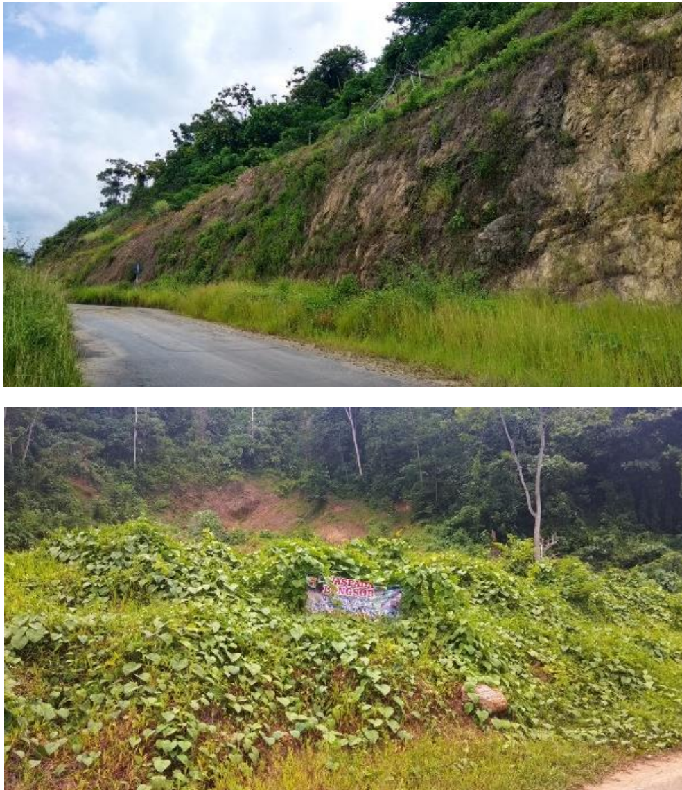
Fig. 3. Landslide with Steep Slope (a and b) in Pekon Tanjung Siom I
