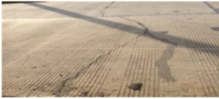
Fig. 4. Single cracks with chain
