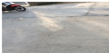
Fig. 3. Single crack lying a cross the rigid pavement with fine cracks
