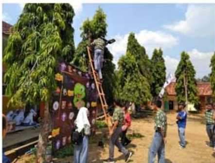
Gambar 9. Instalasi Penerangan Listrik tenaga surya off-grid
