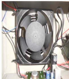
Figure 5a. Cooling fan before modification
