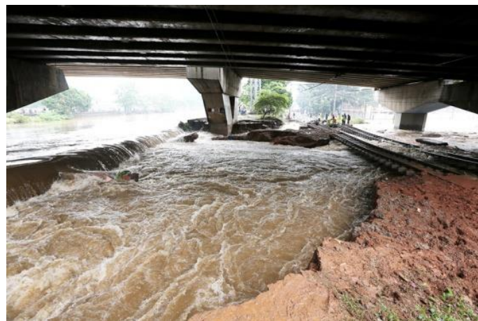
Figure 3. Ballast layers and subgrade washed out (The Jakarta post, 2013)
