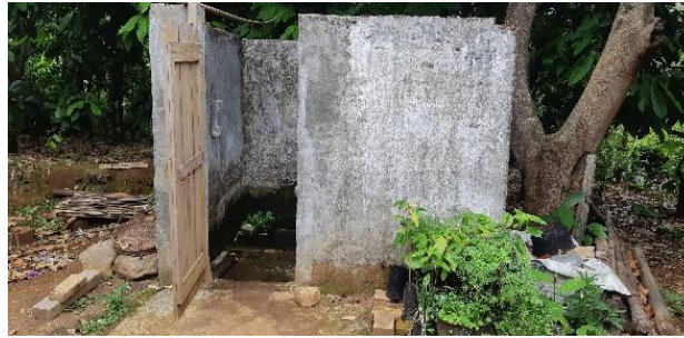
Gambar 7. Kondisi toilet KLS Figure 7. Toilet condition of KLS
