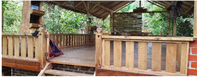
Gambar 6. Kondisi gazebo KLS Figure 6. Gazebo condition of KLS
