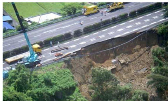
Figure-1. Tomei expressway fault after Surugawan earthquake in 2009 ( http://mtokyoblog.blogspot.jp/2009_08_01_archive.html ).
