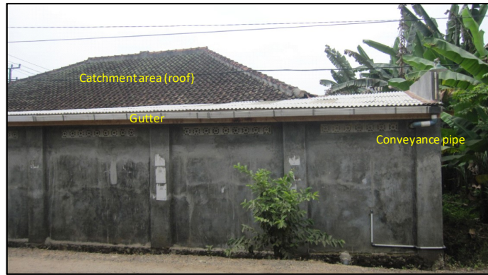
Figure 5. Catchment area (roof), gutter, and conveyance pipe
