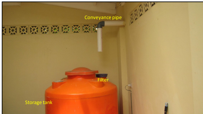
Figure 7. Storage tank, filter, and conveyance pipe
